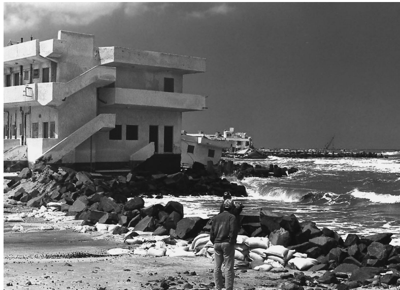
Fig. 6. Field photograph showing severe erosion affecting buildings in Baltim.
